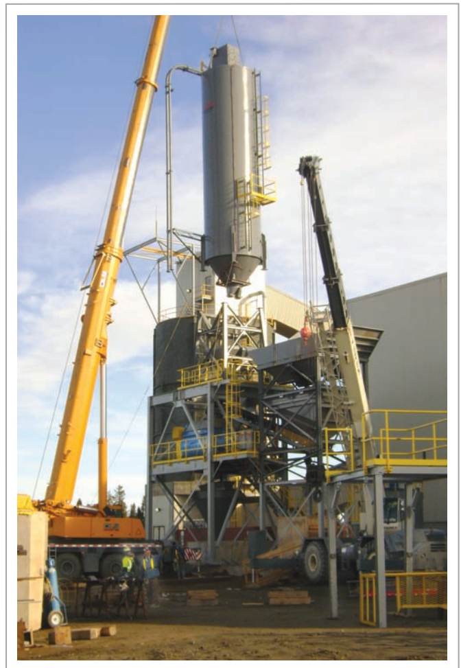
300-Ton DLB Crane working with 65-Ton DLB crane places 20-Ton Silo on top of CaNickel Paste Plant, November 2011
